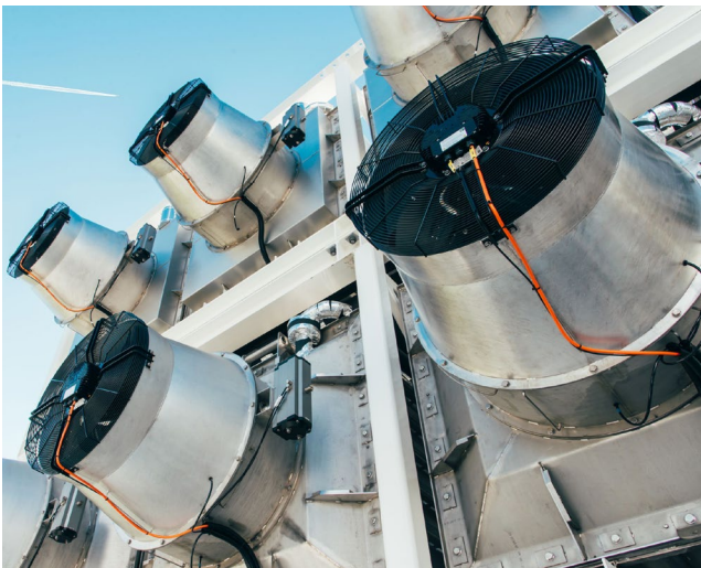
Die Climeworks-DAC-Anlage in Hinwil
